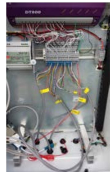
Data logger connections
