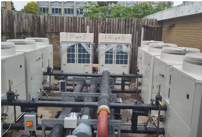
Haldane Building, air source heat pump
