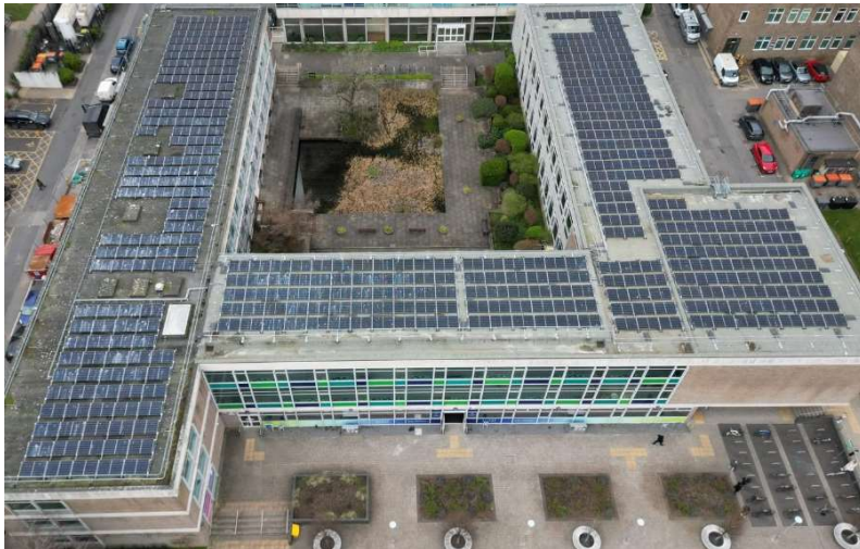
Glyndwr solar array, part of 1800 panel install
