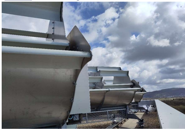
CISM Building 3x Crossflow wind turbines
