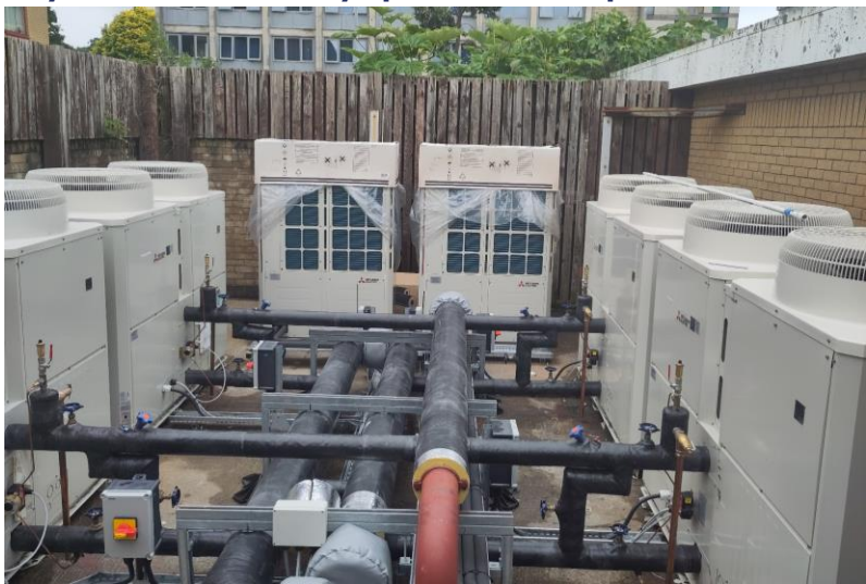
Haldane Building, air source heat pump
